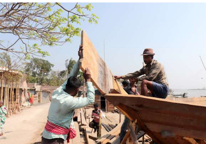
Figure 12 : Young people are also engaged with boat building in Ichhamati river, Basirhat, North 24 Parganas. Malaysian Teak and other imported woods are widely used due to availability and low price.
